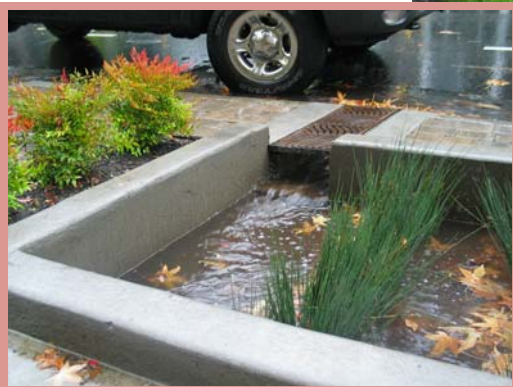
Figure 6.28 - SW 12th Ave., Portland, Oregon - Landscaped Stormwater Planters (ASLA Photo)
